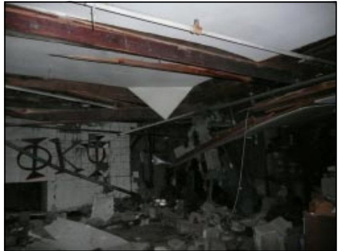
This photo shows extensive damage in the chapter house basement. Ceiling beams are split and the cinder block wall is partially destroyed. The boiler was in a room at the right.
